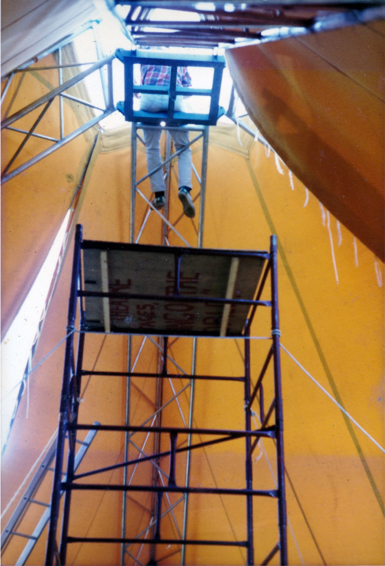
Fig. 4. Erecting the pyramid theatre. The legs are assembled, the tops then raised up onto the scaffold tower where they are fixed to the (very heavy!) steel top piece. The legs are then moved inwards to raise the assembly to full height, and joined by rigging wires to make the structure secure. Then someone (in this case Bill Scott) has to go up there to finish off. Photo by the author (CC BY-NC 4.0).
