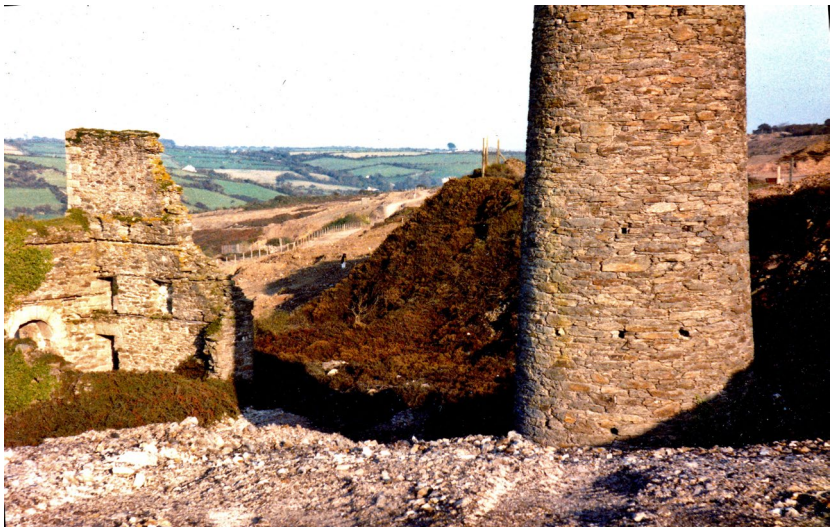
Fig. 8. Granite mine buildings on the slopes above Wheal Maid, 1984. The Carnon Valley can be seen in the distance. Photo by the author (CC BY-NC 4.0).
