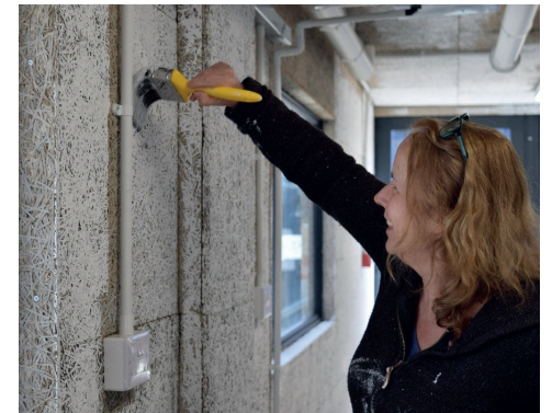
ABOVE: Artist Sinead O'Connor putting the first coat of paint on her new studio at Krowji
